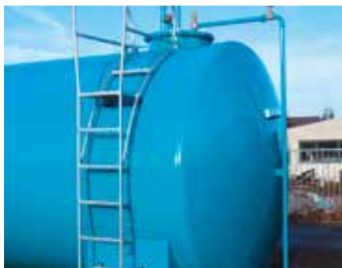
Diesel tank with platform and suction line
